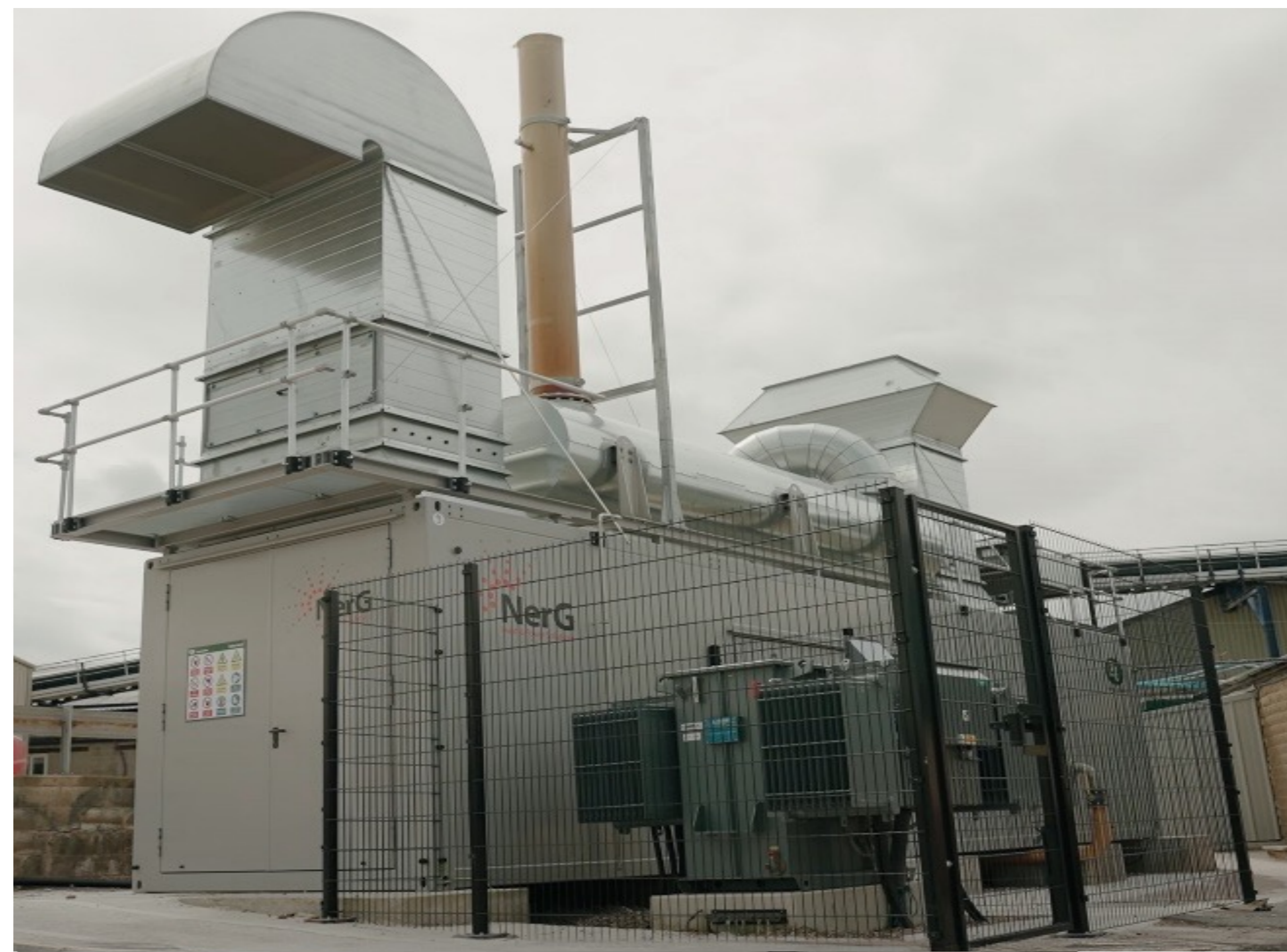
Credit: Naylor Industries - Combined Heat & Power plant
