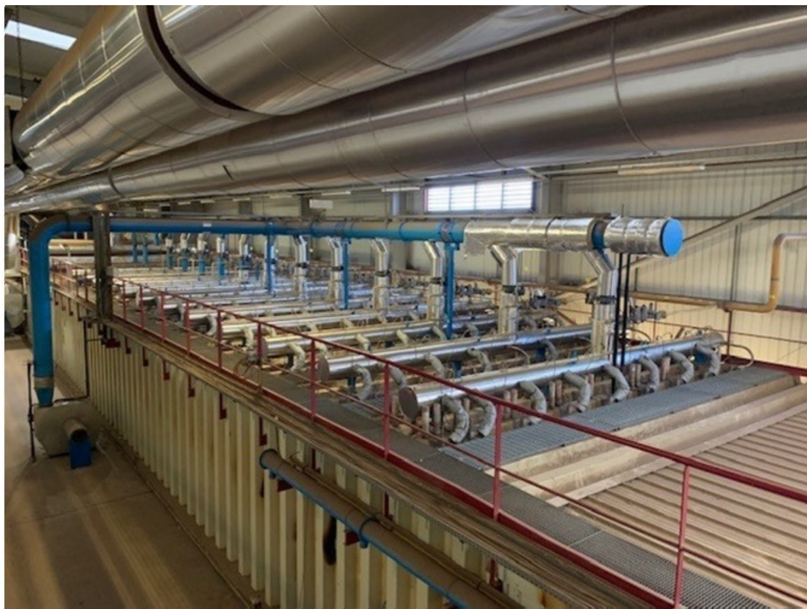
Credit: Wienerberger - Heat Recovery System at Broomfleet factory
